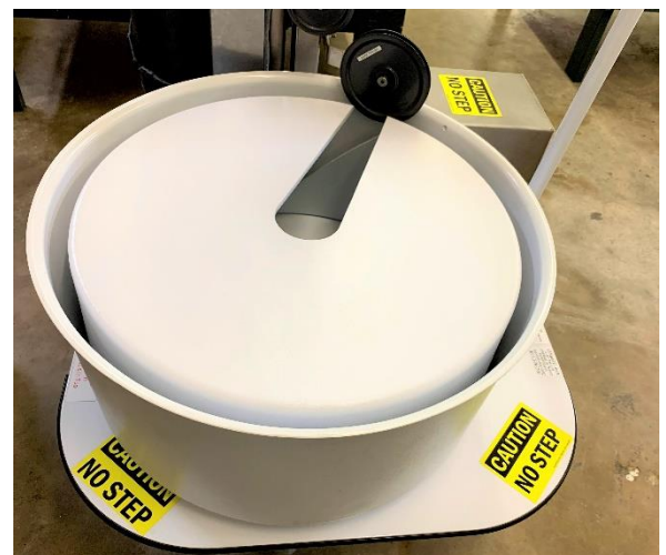
Figure 18 No Step Warning Labels
